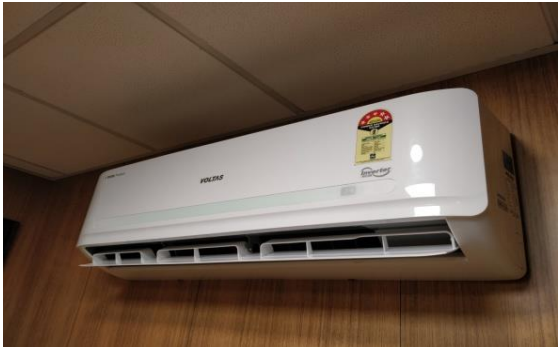
Energy efficient inverter type AC units
